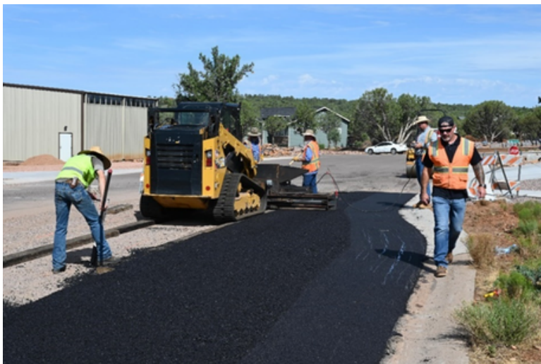
Tim Ryden inspects the repair as Shawn and Vince clean the intake for another round of asphalt. Tuger rakes out the fines and preps the patch for compaction.
