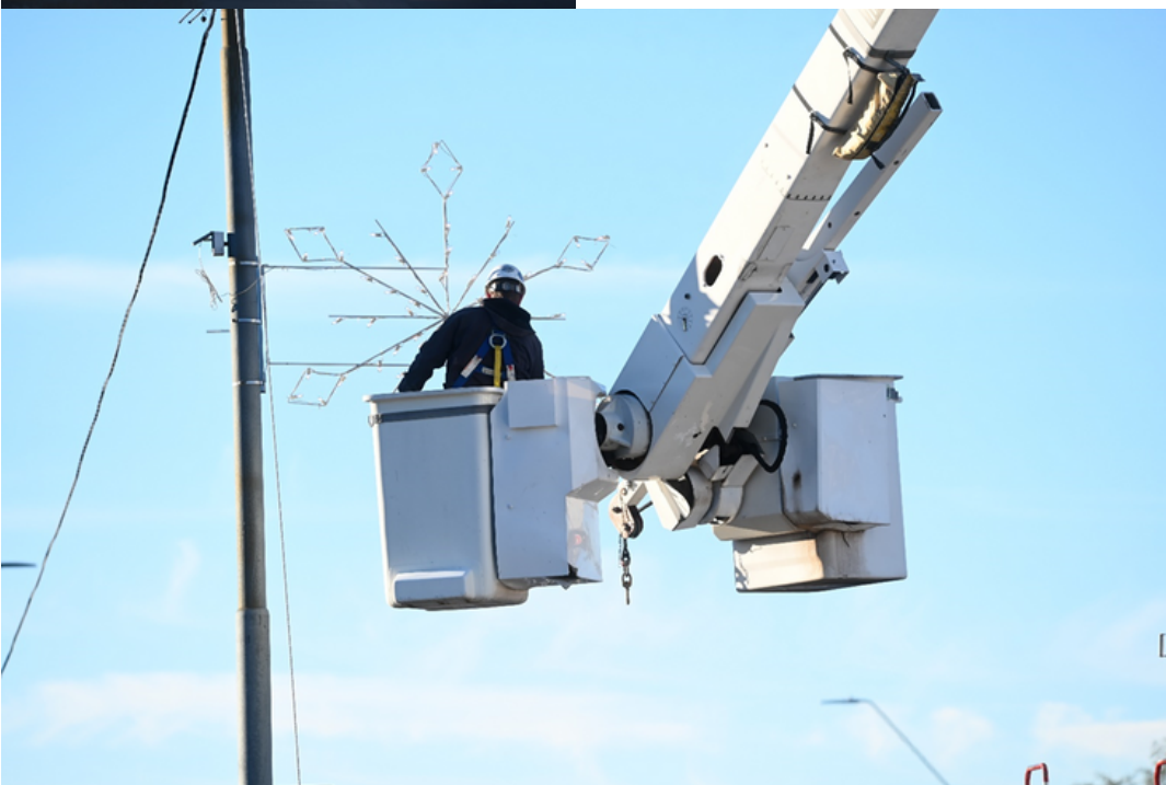
Shane handles a snowflake as he and the crew installed over 100 marquees in a two day period.
