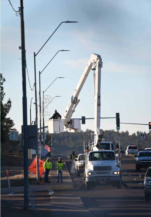
KC, Houston, and The Ang manage traffic and situational awareness as Shane installs a Decorative Marquee on Beeline Highway.
