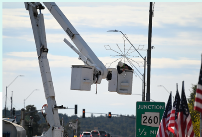
Wyatt hooks and powers one of 103 individual LED candelabras along ADOT's primary routes of travel Highways 87 and 260.
