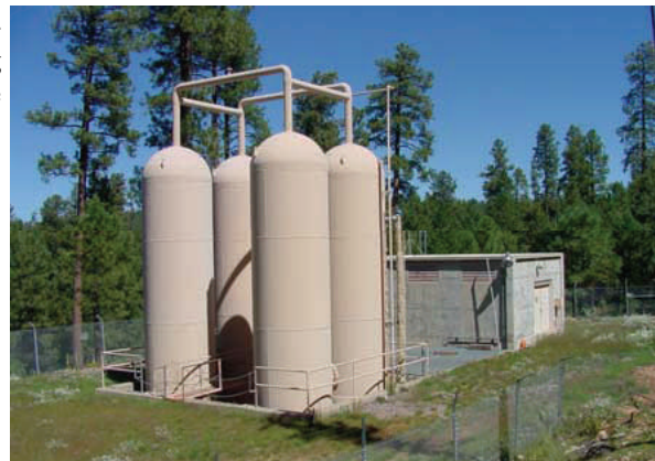
C.C. Cragin Pumping Station
