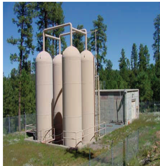
C.C. Cragin Pumping Station
